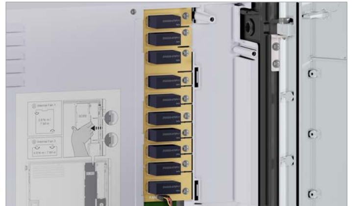
Fig. 4.11: View of the DC surge protection devices with the cover removed
